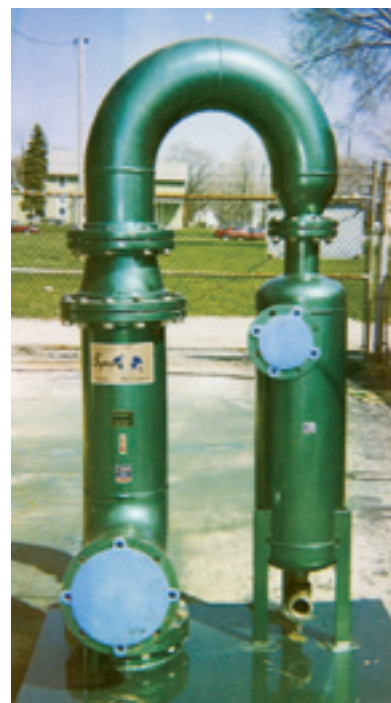
Fig. 9 — Magnetic water conditioning installation.
